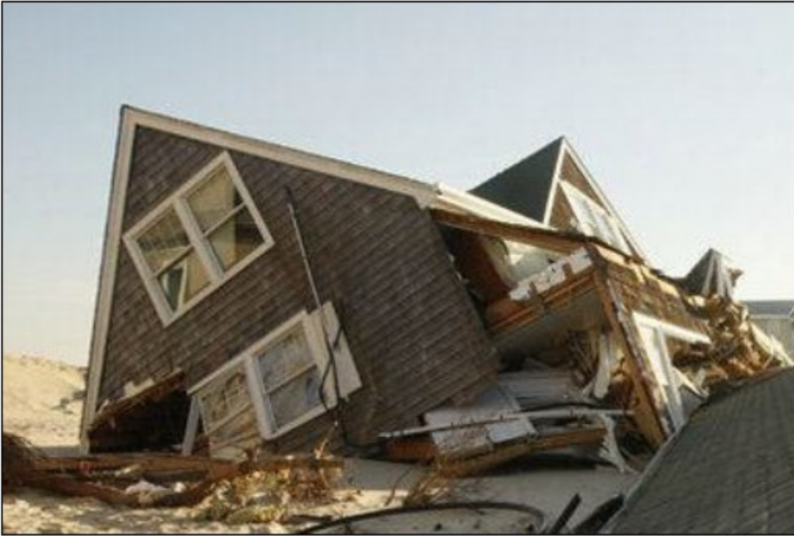
Image #7: The above example photo illustrates a building that is off of its foundation.
